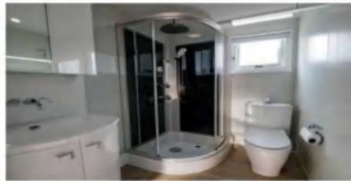
Bathroom with toilet, basin, faucet, cabinet, mirror and shower room
